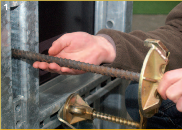
1 Install Rapid Locking Bar with welded counter plate at the first formwork panel.
